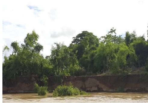
Plate 4: Bank erosion at Kyaukye Village (27.6.17)
